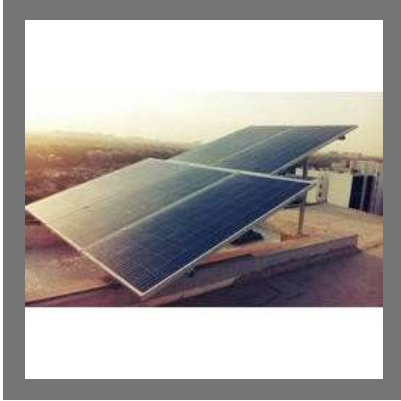
Home Solar Rooftop System
