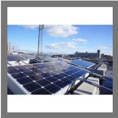
Industrial Solar Power Rooftop Systems
