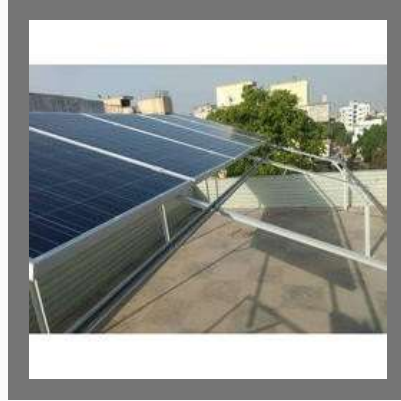
5 KW Solar Rooftop System
