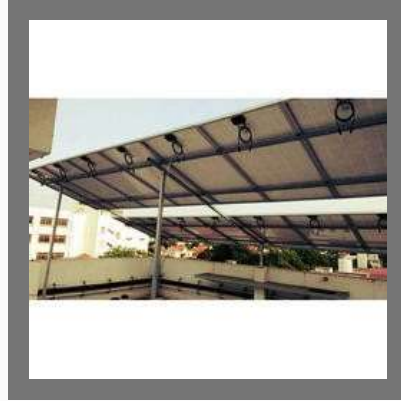
Solar Panel Mounting Structure
