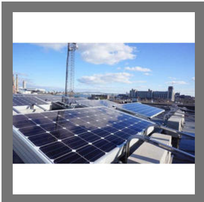
Industrial Solar Power Rooftop Systems
